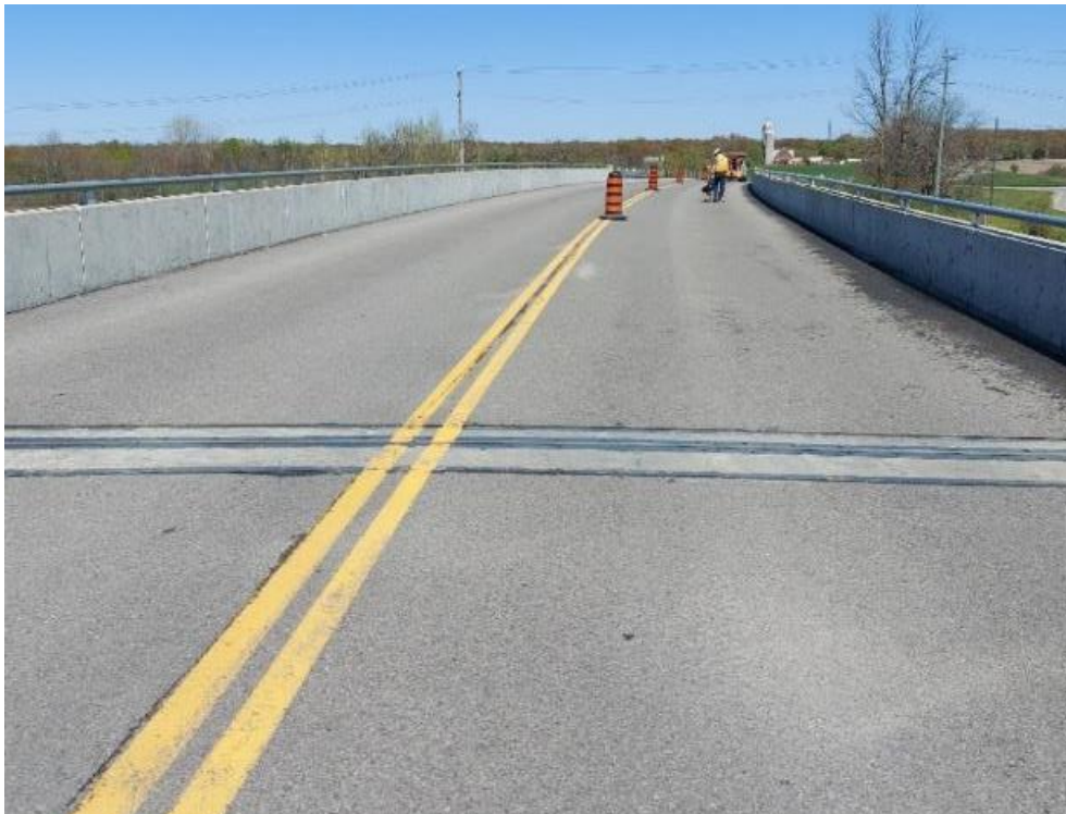
Photograph 6: Bridge No. 16-165 – Highway 401 Blue Church Road Underpass. General view looking north along the bridge.
