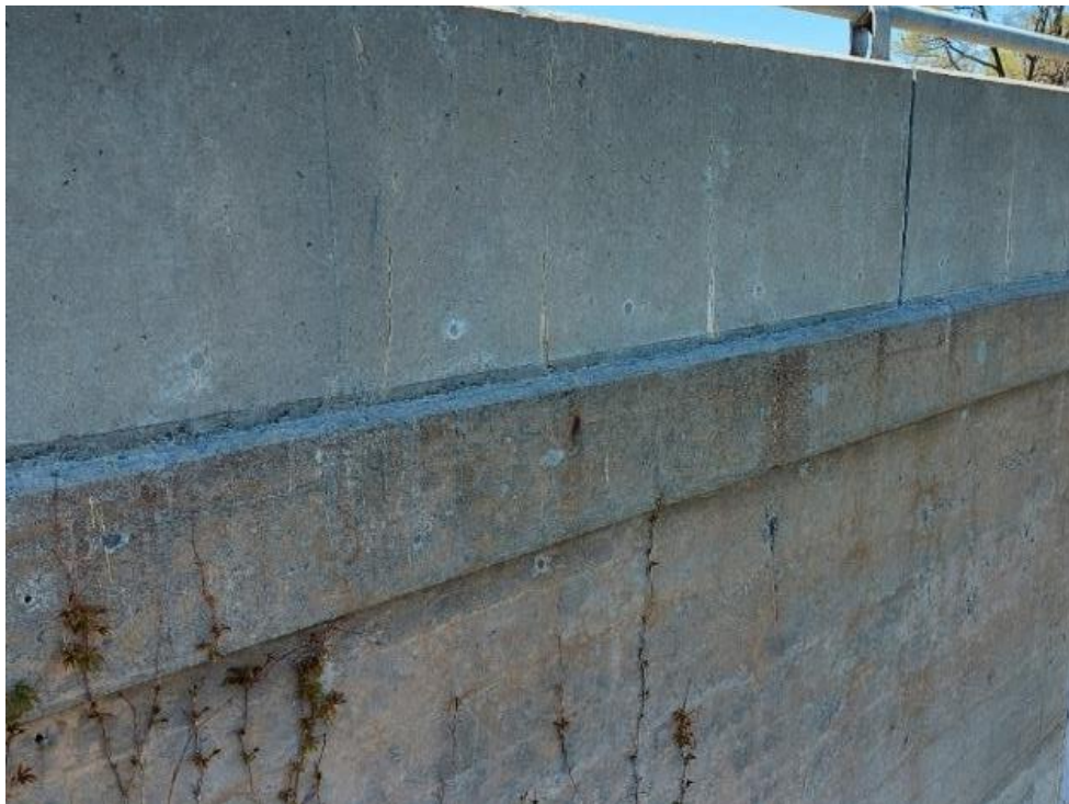
Photograph 18: Bridge No. 16-128 – Highway 401 Edward Street Interchange. View of the east side of the bridge with no date stamp present.
