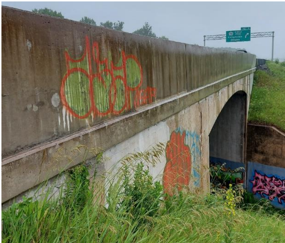
Photograph 24: Bridge No. 16-129 – Highway 401 CPR Overhead. View of the south side of the bridge with no date stamp present.
