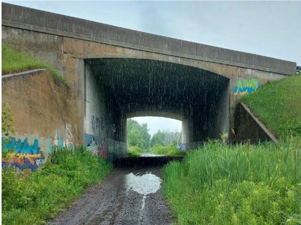
Photograph 25: Bridge No. 16-129 – Highway 401 CPR Overhead. General view of underside of the bridge along former CNR right of way.
