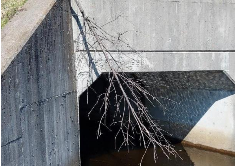
Photograph 57: Structural Culvert 16-259/C – Highway 401 W-416N Ramp Culvert. View of culvert stamp with construction date along the east side of the culvert. Culvert stamped 16-259-1998.
