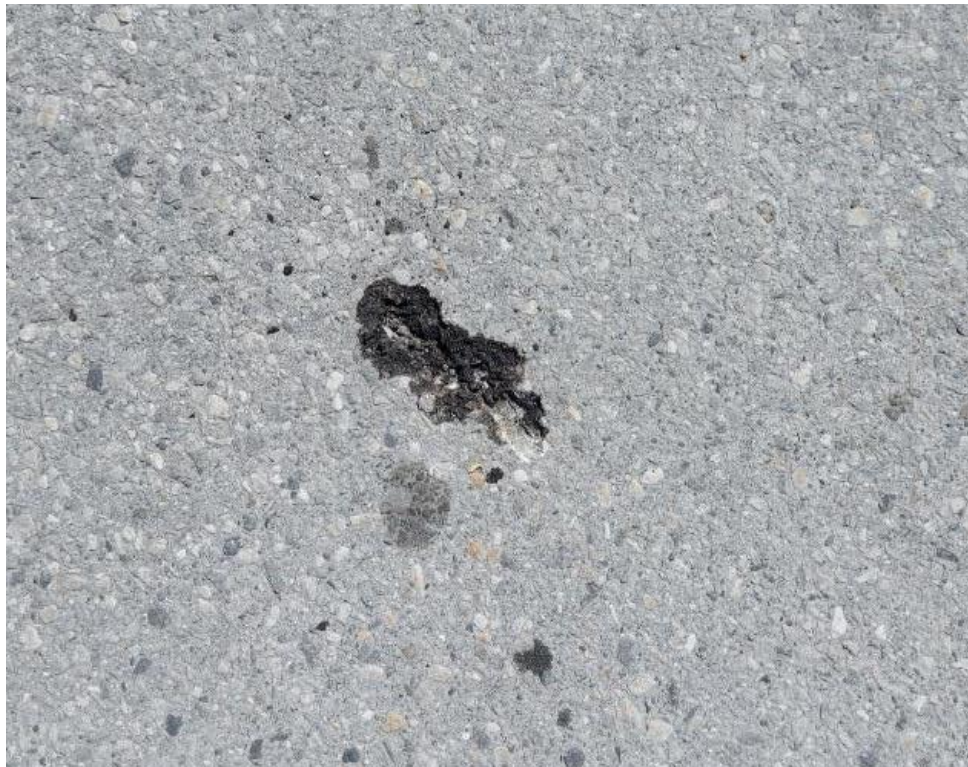
Photograph 22: Bridge No. 16-128 – Highway 401 Edward Street Interchange. View of bulk asphalt sample 16-128-ASP-01A along top side of the bridge. All bulk samples collected from the Site found not to contain asbestos.
