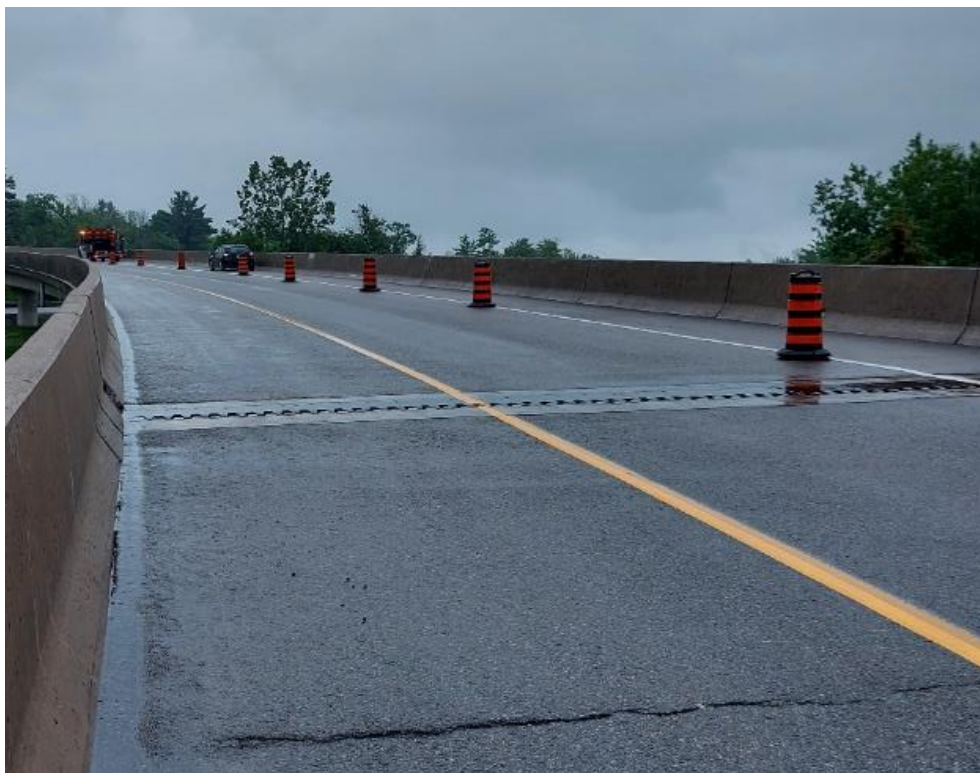
Photograph 32: Bridge No. 16-308 – Highway 401 Southbound Connector N-E. General view looking south along the bridge.
