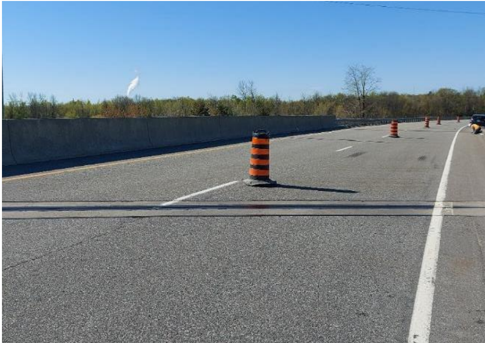
Photograph 27: Bridge No. 16-307 – Highway 401 Cedar Grove Road Overpass. General view looking south along the bridge.
