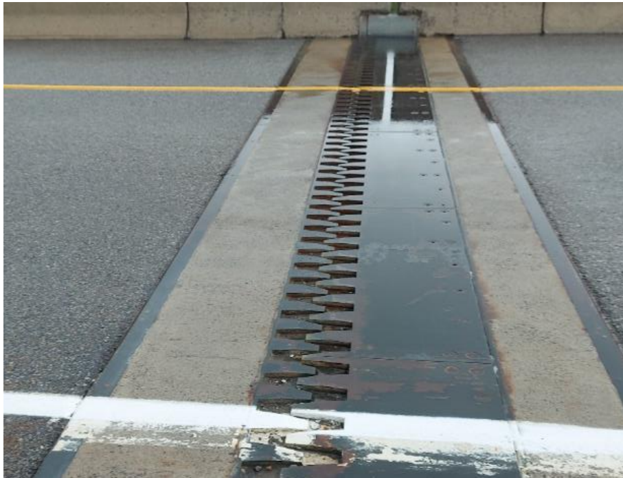
Photograph 35: Bridge No. 16-308 – Highway 401 Southbound Connector N-E. View of bridge deck expansion joint along the north side of the bridge.
