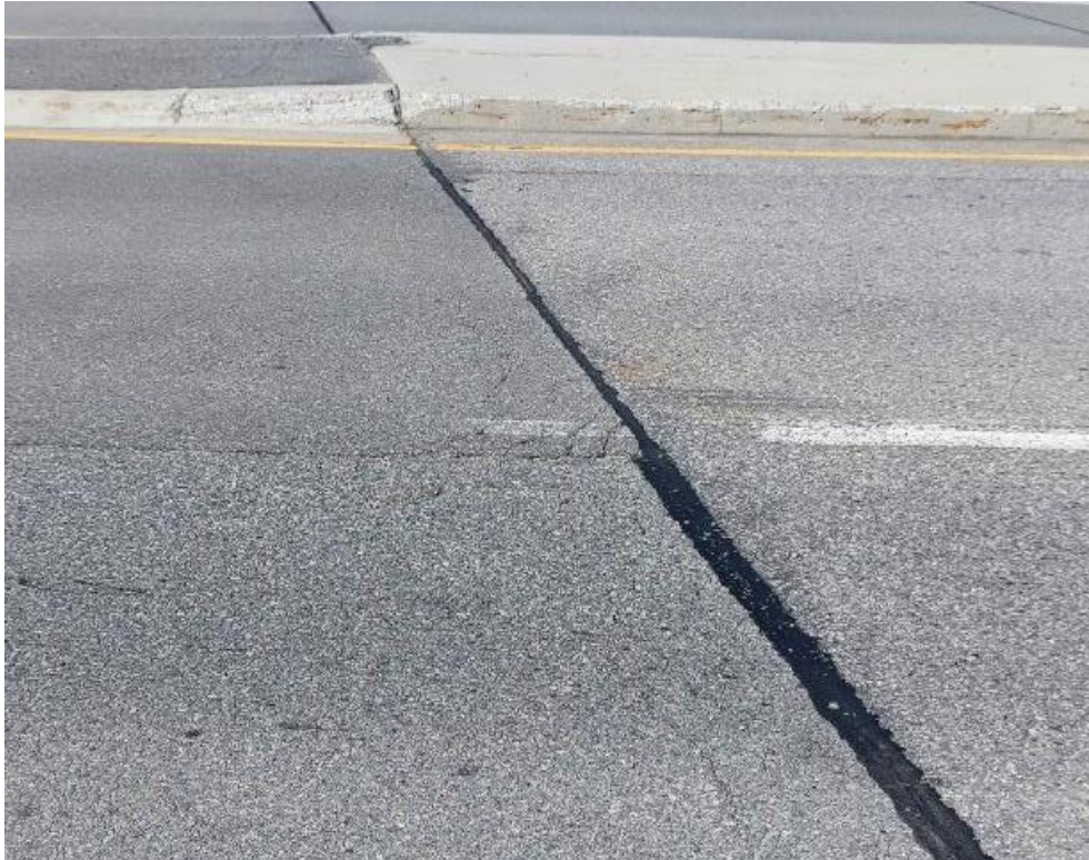
Photograph 49: Bridge No. 16-131 – Highway 16 CNR Overhead. View of bridge boundary along the south side of the bridge.
