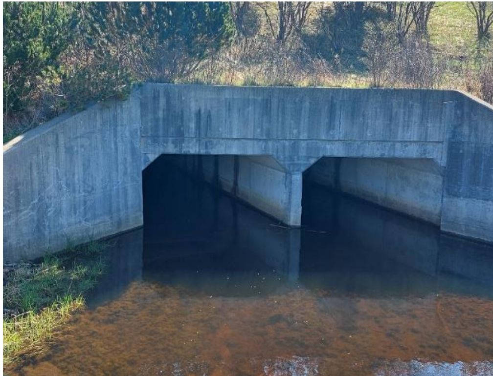
Photograph 58: Structural Culvert 16-259/C – Highway 401 W-416N Ramp Culvert. General view of structural culvert along the north side of Highway 416 south abutment.
