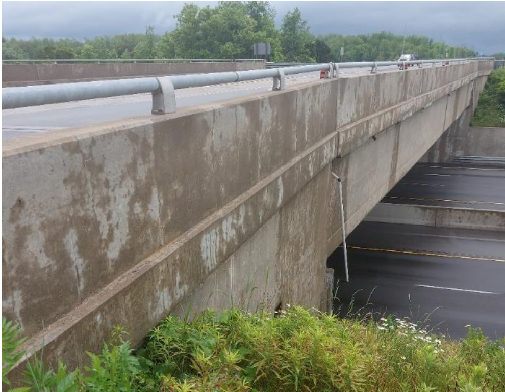
Photograph 45: Bridge No. 16-130-Highway 16 U/P. View of concrete barrier wall along west side of bridge with single tube metal railing.
