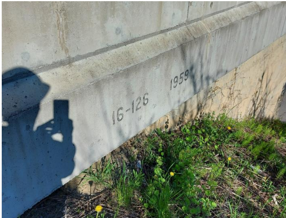
Photograph 2: Bridge No. 16-126 – Highway 401 Maitland Road Interchange. View of bridge stamp with construction date along the east side of the bridge. Bridge stamped 16-126-1959.
