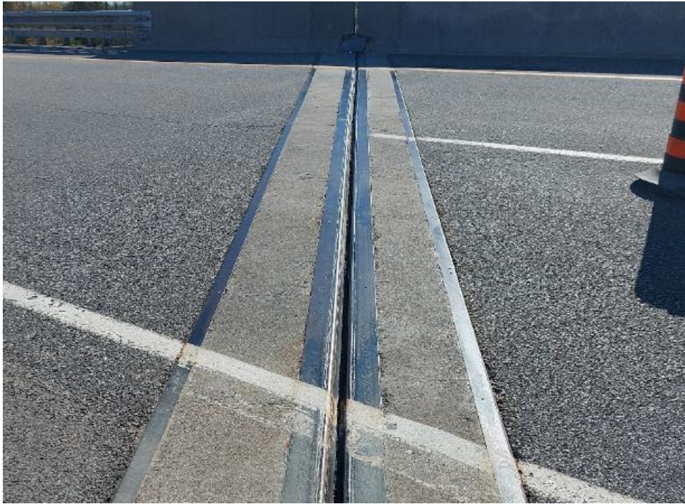
Photograph 29: Bridge No. 16-307 – Highway 401 Cedar Grove Road Overpass. View of a bridge deck expansion joint along the north side of the bridge.
