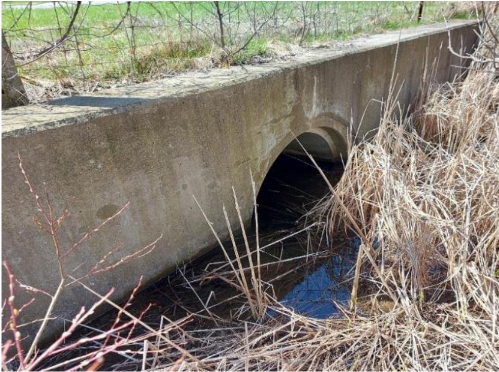
Photograph 63: Additional culvert at Project Site: View of additional culvert located along the north side of Cedar Grove Road east of the bridge Site 16-307. Culvert was not stamped with any identification or construction date.
