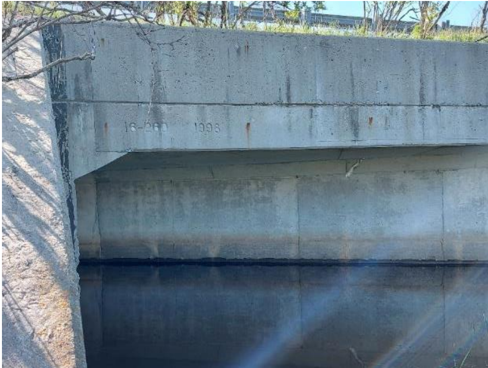
Photograph 59: Structural Culvert 16-260/C – Highway 401 W-401W Ramp Culvert. General view of structural culvert along the south side Highway 416 south abutment. Culvert stamped 16-260-1998.
