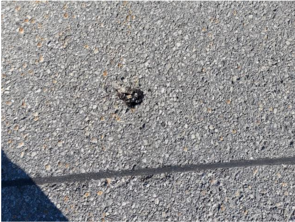
Photograph 5: Bridge No. 16-126 – Highway 401 Maitland Road Interchange. View of bulk asphalt sample 16-126-ASP-01A along top side of the bridge. All bulk samples collected from the Site found not to contain asbestos.
