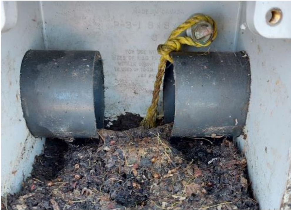
Photograph 41: Bridge No. 16-306 – Highway 401/416 W-N Ramp. View of conduit hatch with PVC piping along the east side of the bridge. The hatch did not contain any electrical wiring.
