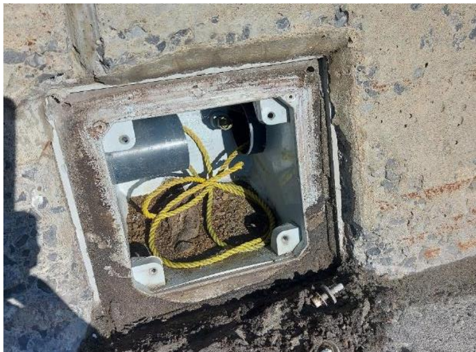
Photograph 30: Bridge No. 16-307 – Highway 401 Cedar Grove Road Overpass. View of conduit hatch with PVC piping along the east side of the bridge. The hatch did not contain any electrical wiring.
