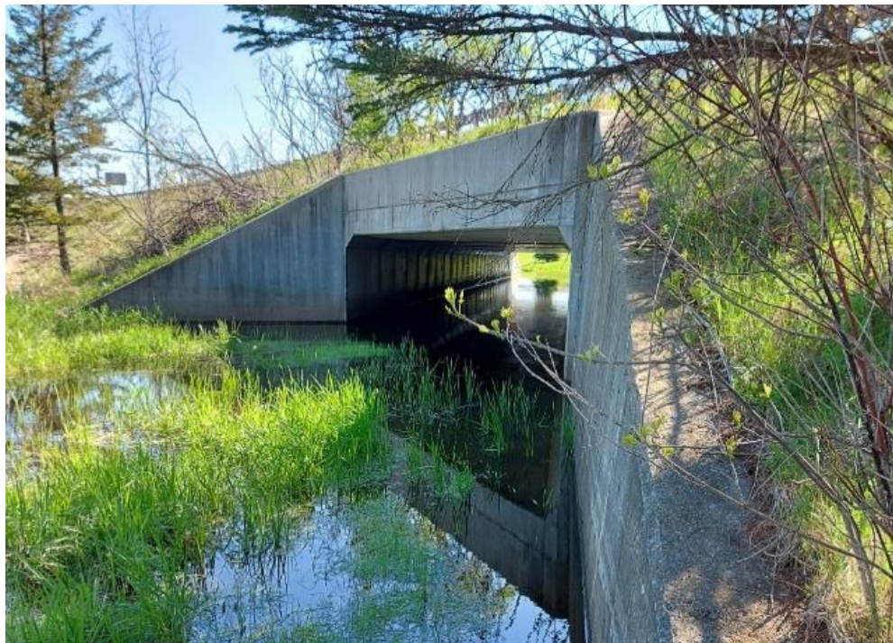
Photograph 60: Structural Culvert 16-260/C – Highway 401 W-401W Ramp Culvert. General view of structural culvert along the north side Highway 416 south abutment Structural
