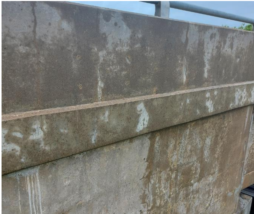
Photograph 44: Bridge No. 16-130-Highway 16 U/P. View of west side of bridge with no date stamp present.
