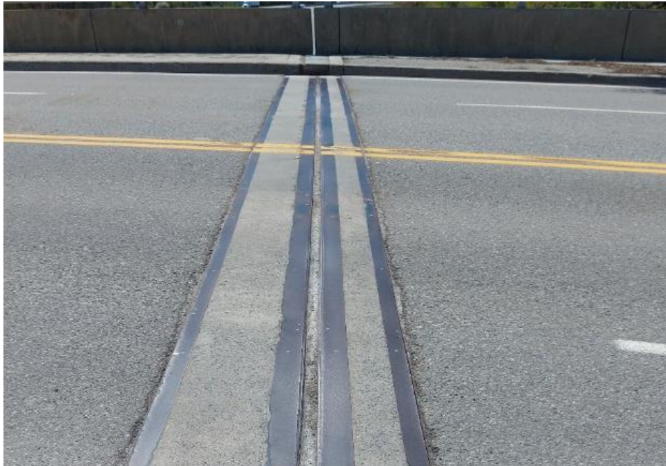
Photograph 21: Bridge No. 16-128 – Highway 401 Edward Street Interchange. View of the bridge deck expansion joint along the north side of the bridge.
