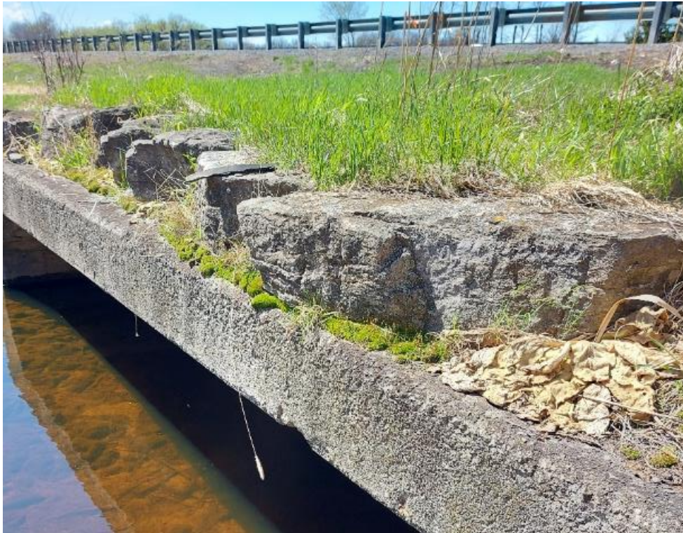
Photograph 55: Structural Culvert 16-250/C – Highway 401 Culvert. General view of single structural culvert along underside of Highway 401 EB/WB Right of Way.
