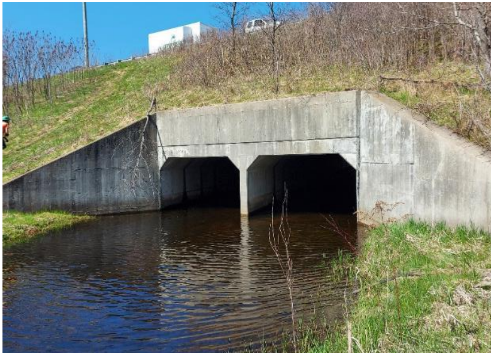
Photograph 56: Structural Culvert 16-259/C – Highway 401 W-416N Ramp Culvert. General view of structural culvert along south side of Highway 416 south abutment.
