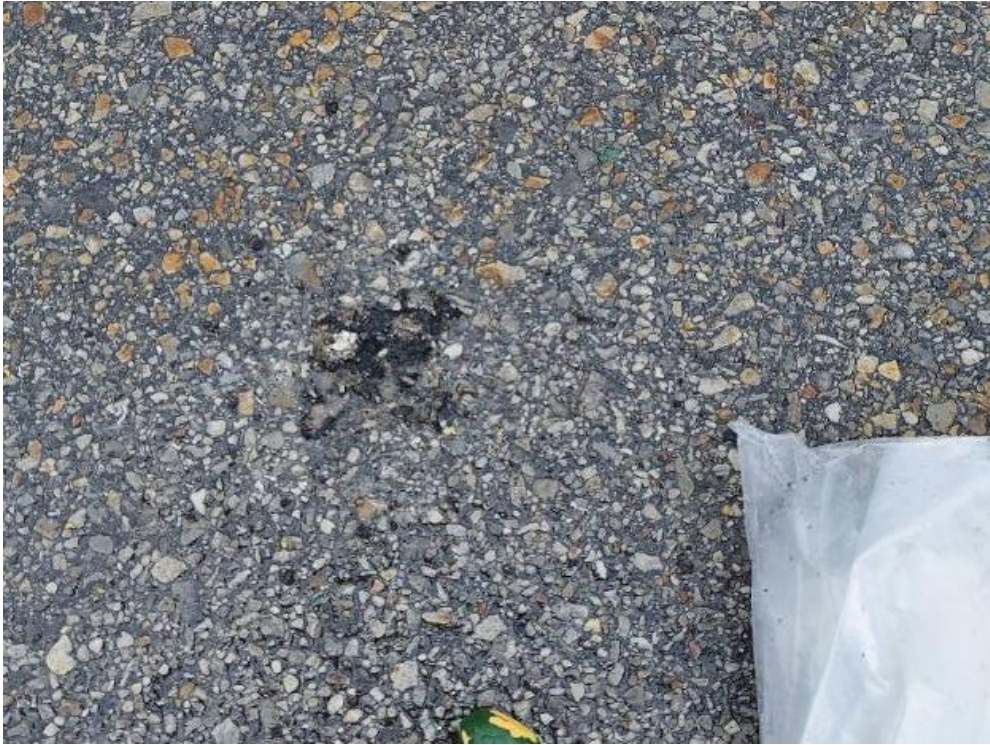
Photograph 37: Bridge No. 16-308 – Highway 401 Southbound Connector N-E. View of bulk asphalt sample 16-308-ASP-01A along top side of the bridge. All bulk samples collected from the Site found not to contain asbestos.
