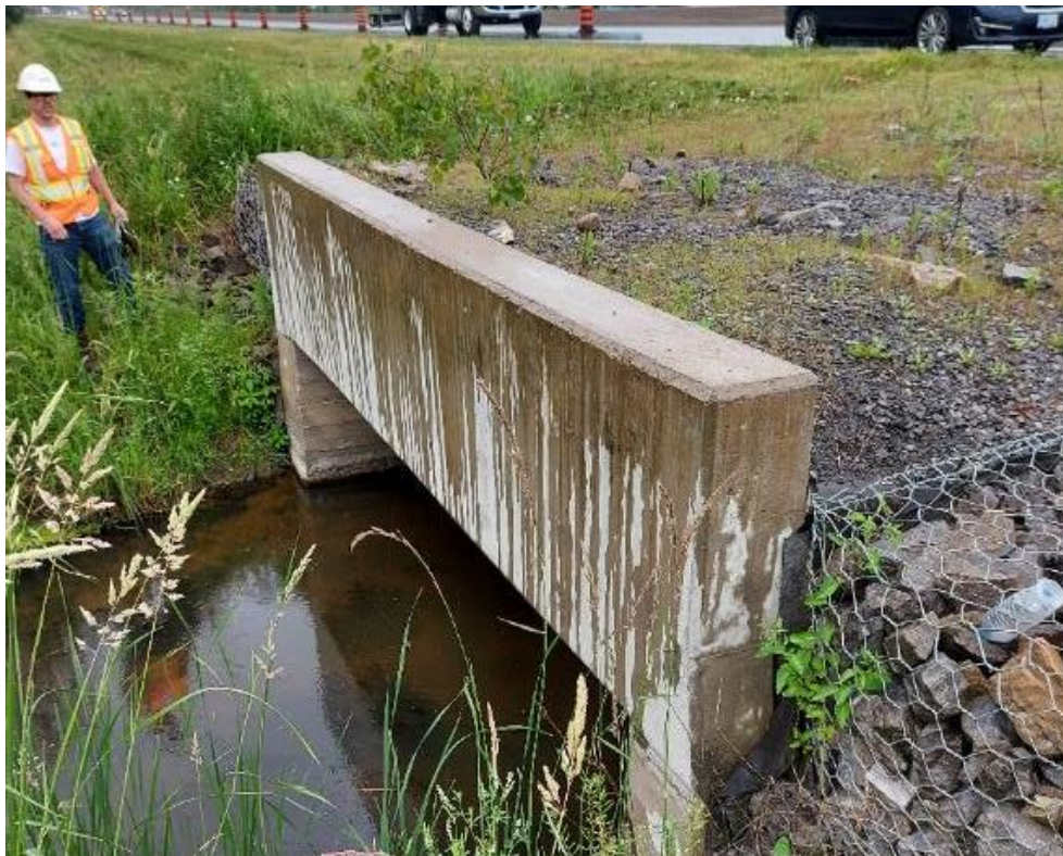
Photograph 52: Structural Culvert 16-239/C – Highway 401 Lemmon’s Creek Culvert. View of culvert along underside of Highway 401 ROW.
