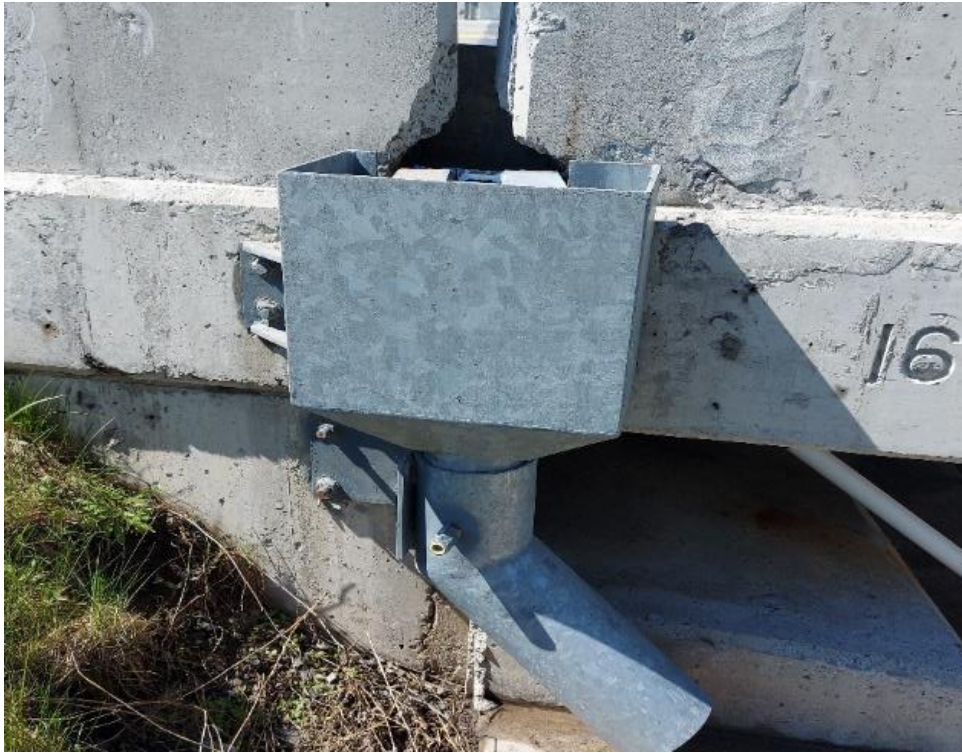
Photograph 9: Bridge No. 16-165 – Highway 401 Blue Church Road Underpass. View of metal surface drain pipe along the east side of the bridge.
