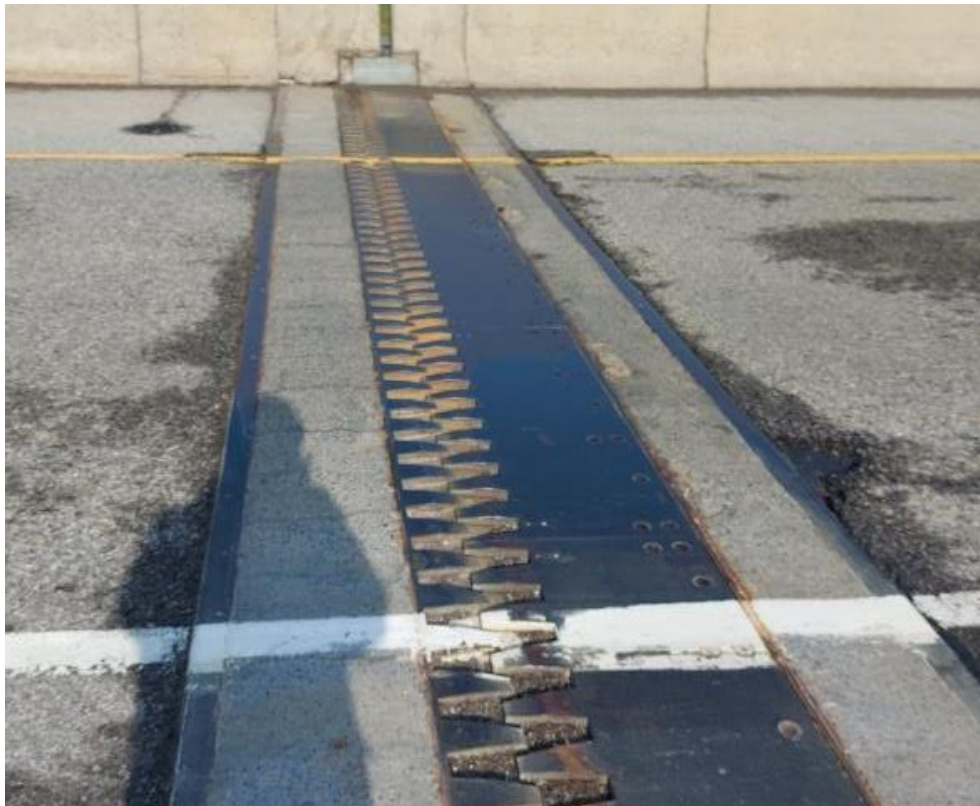
Photograph 40: Bridge No. 16-306 – Highway 401/416 W-N Ramp. View of bridge deck expansion joint along the north side of the bridge.
