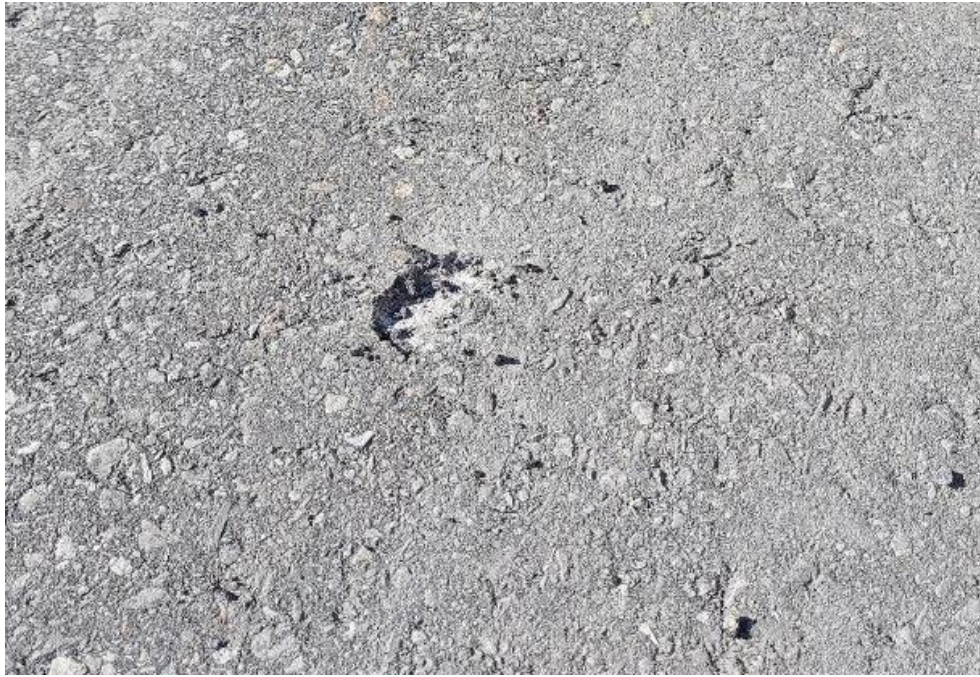
Photograph 31: Bridge No. 16-307 – Highway 401 Cedar Grove Road Overpass. View of bulk asphalt sample 16-307-ASP-01A along top side of the bridge. All bulk samples collected from the Site found not to contain asbestos.
