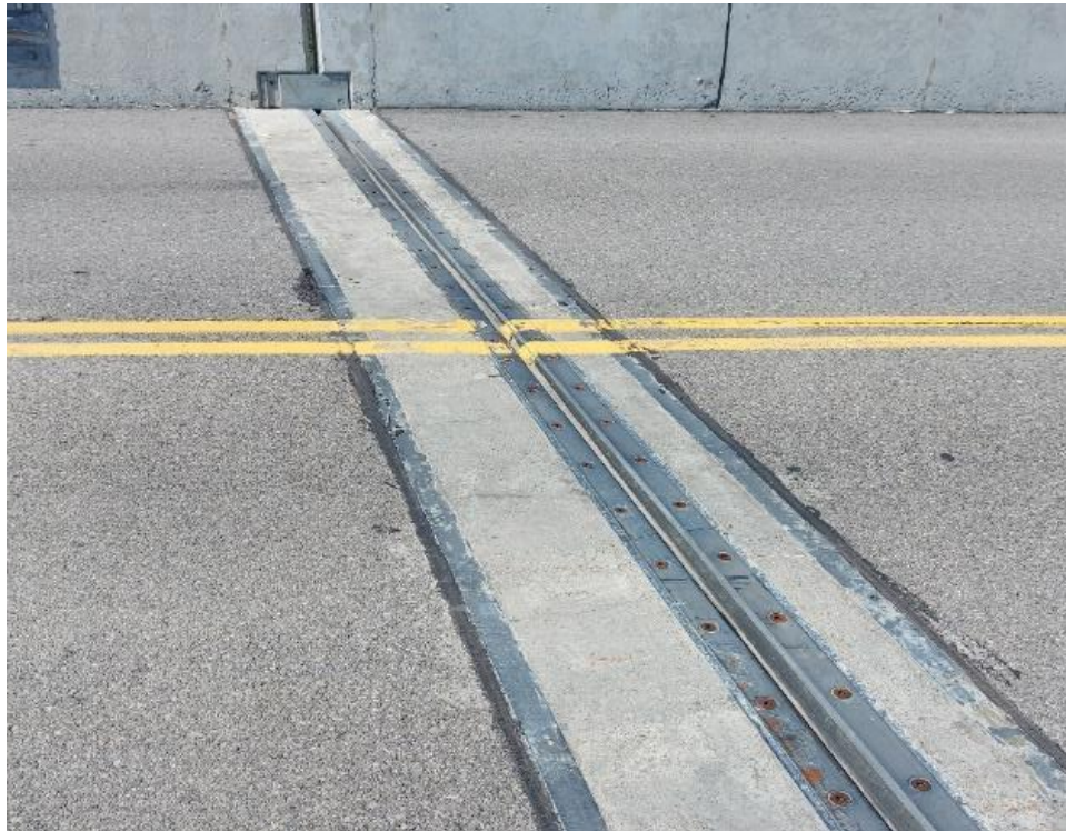
Photograph 8: Bridge No. 16-165 – Highway 401 Blue Church Road Underpass. View of bridge deck expansion joint along the south side of the bridge.
