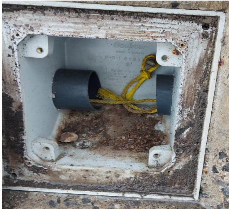
Photograph 36: Bridge No. 16-308 – Highway 401 Southbound Connector N-E. View of conduit hatch with PVC piping along the east side of the bridge. The hatch did not contain any electrical wiring.
