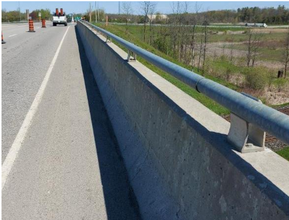
Photograph 50: Bridge No. 16-131 – Highway 16 CNR Overhead. View of concrete barrier wall along the east side of the bridge.
