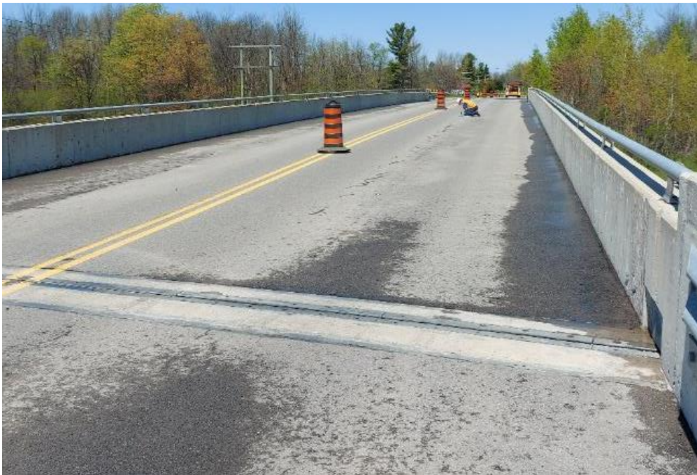
Photograph 12: Bridge No. 16-166 – Highway 401 Merwin Lane Underpass. General view looking north along the bridge.
