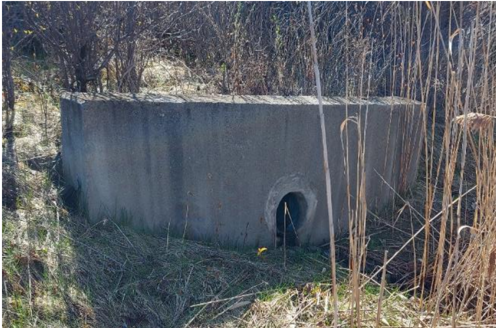
Photograph 61: Additional culvert at Project Site: View of additional culvert located along the north side of Highway 416 south abutment immediately west of culvert 16-259. The south portion of the additional culvert could not be located by AECOM. Culvert was not stamped with any identification or construction date.
