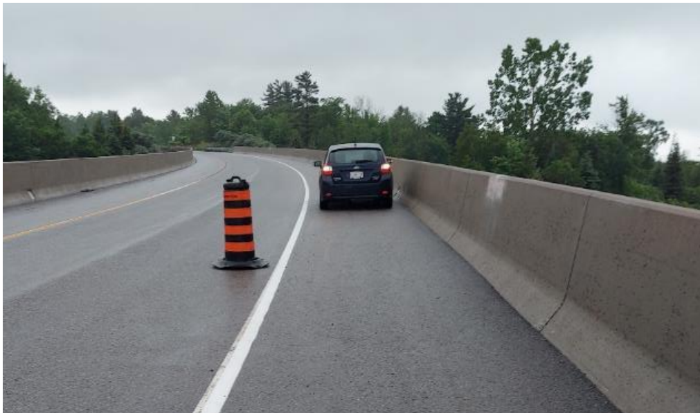
Photograph 34: Bridge No. 16-308 – Highway 401 Southbound Connector N-E. View of concrete barrier wall along The east side of the bridge.
