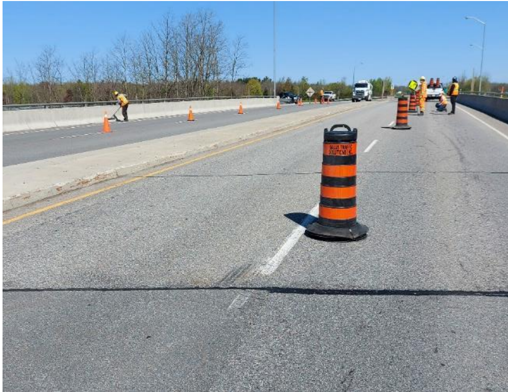
Photograph 47: Bridge No. 16-131 – Highway 16 CNR Overhead. General view looking north along the bridge.
