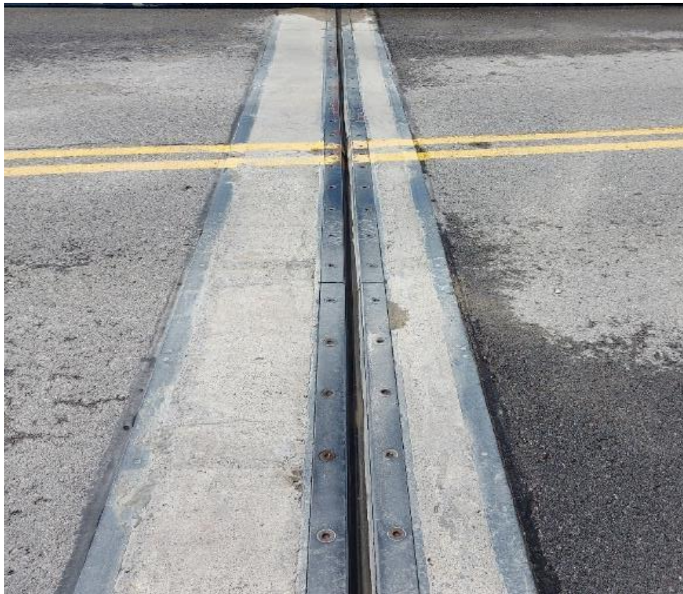
Photograph 14: Bridge No. 16-166 – Highway 401 Merwin Lane Underpass. View of bridge deck expansion joint along the south side of the bridge.
