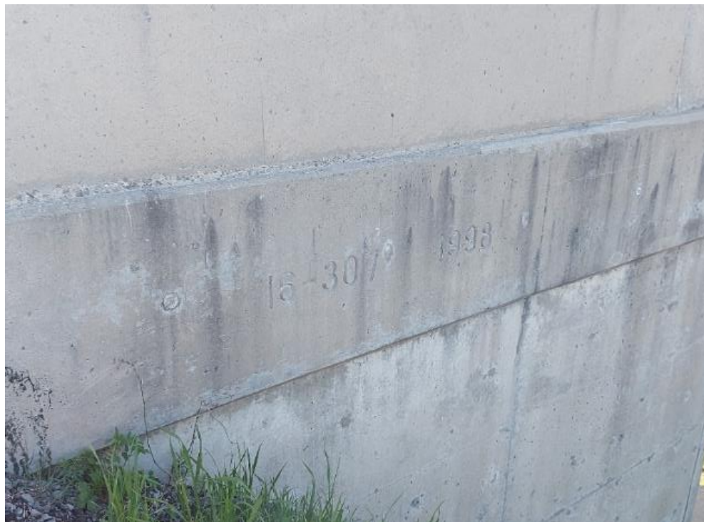
Photograph 28: Bridge No. 16-307 – Highway 401 Cedar Grove Road Overpass. View of bridge stamp with construction date along the west side of the bridge. Bridge stamped 16-307-1998.
