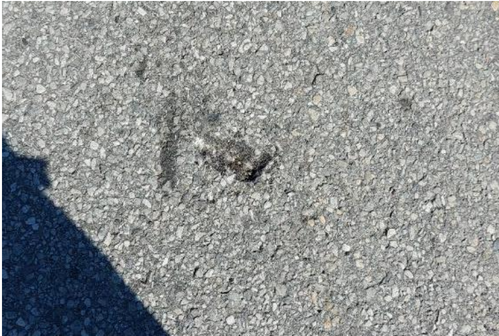
Photograph 51: Bridge No. 16-131 – Highway 16 CNR Overhead. View of bulk asphalt sample 16-131-ASP-01A along top side of the bridge. All bulk samples collected from the Site found not to contain asbestos.
