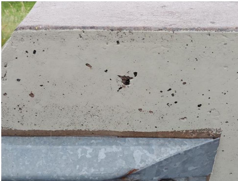
Photograph 26: Bridge No. 16-129 – Highway 401 CPR Overhead. View of paint sample from concrete barrier wall along the south side of the bridge. Paint sample 16-129-PT-01 contained <10 ppm of lead.
