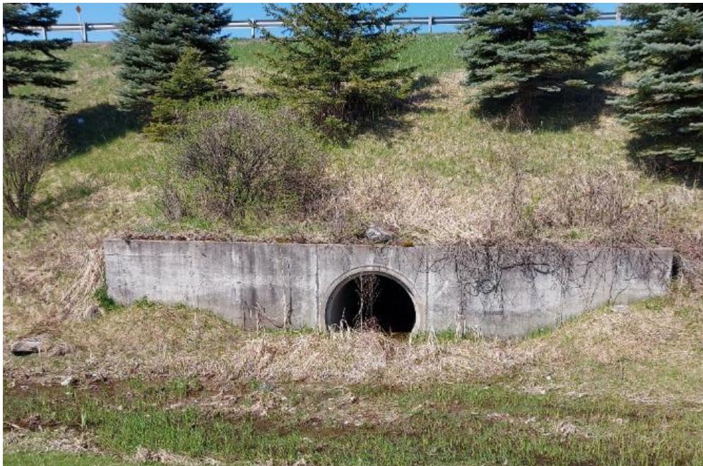
Photograph 62: Additional culvert at Project Site: View of additional culvert located along the south side of Highway 416 north abutment immediately north of bridge Site 16-307. Culvert was not stamped with any identification or construction date.
