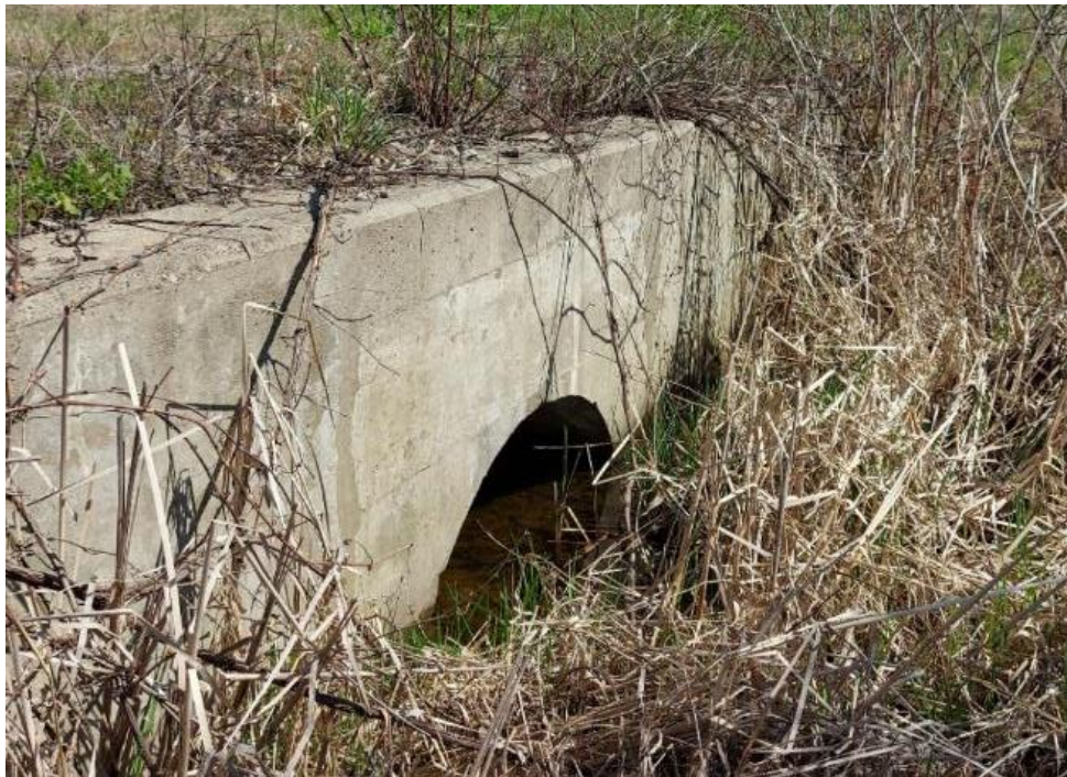
Photograph 64: Additional culvert at Project Site: View of additional culvert located along the south side of Cedar Grove Road east of the bridge Site 16-307. Culvert was not stamped with any identification or construction date.
