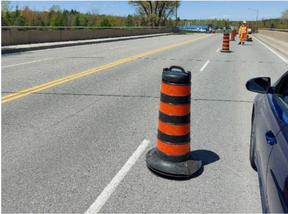
Photograph 17: Bridge No. 16-128 – Highway 401 Edward Street Interchange. General view looking north along the bridge.
