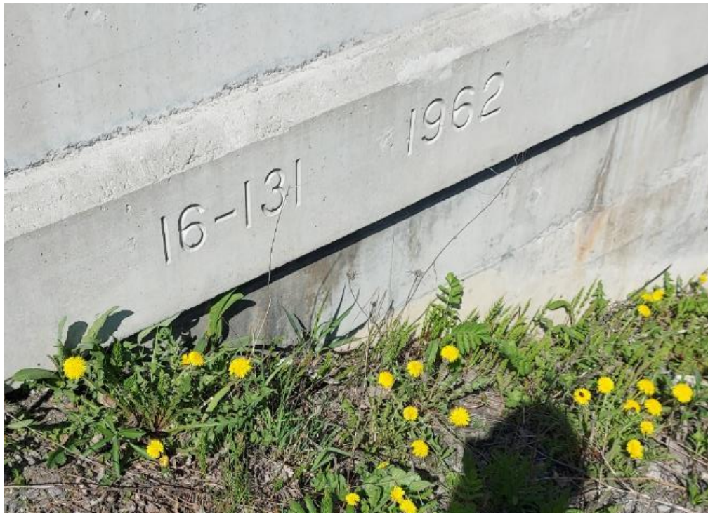
Photograph 48: Bridge No. 16-131 – Highway 16 CNR Overhead. View of bridge stamp with construction date along the east side of the bridge. Bridge stamped 16-131-1962.
