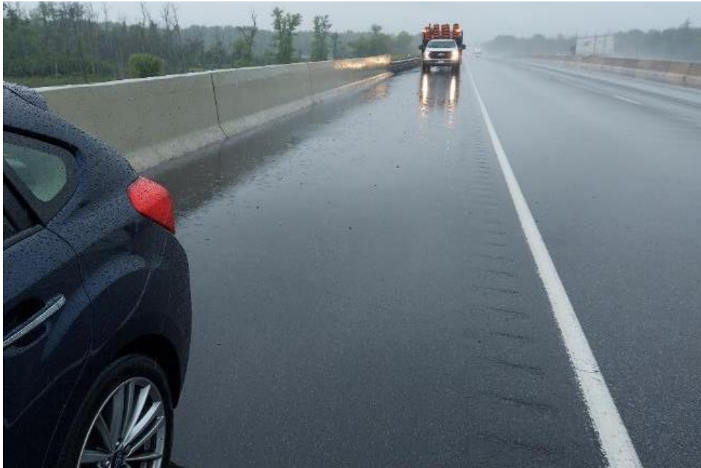
Photograph 23: Bridge No. 16-129 – Highway 401 CPR Overhead. General view looking west along the bridge.
