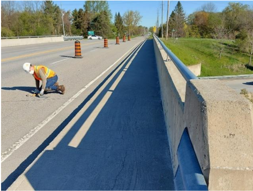
Photograph 3: Bridge No. 16-126 – Highway 401 Maitland Road Interchange. View of concrete barrier wall along the east side of the bridge.
